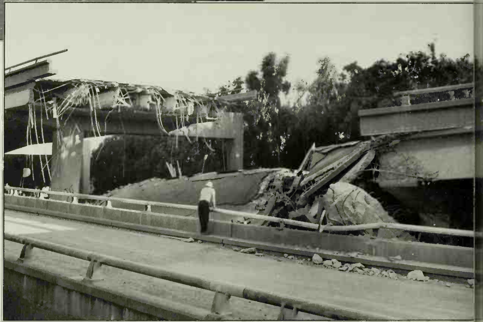
The collapsed Cypress Structure along the Nimitz Freeway, Oakland, after the earthquake of October 17, 1989. Photograph by Steve Ringman. Courtesy San Francisco Chronicle
